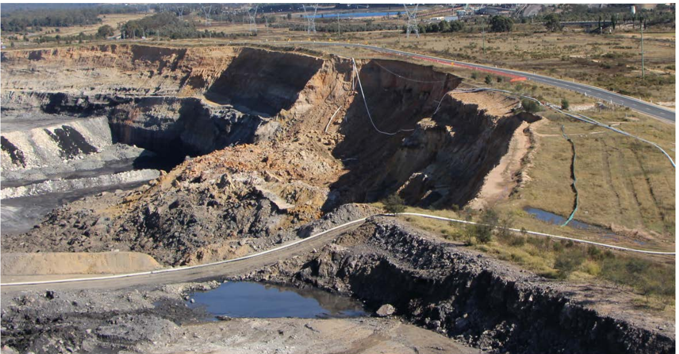
Figure 1: Northern highwall adjacent to Ulan-Wollar Road showing the failure and barricading after the incident. Photographs taken by Moolarben Coal Operations.
