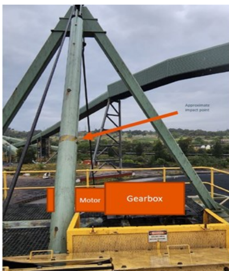
Figure 1: Reclaimer motor and gearbox
