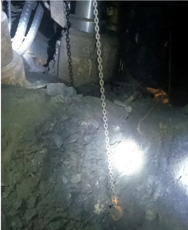
Figure 7: Chain hoist to remove relay bar pin on longwall tailgate roof support
