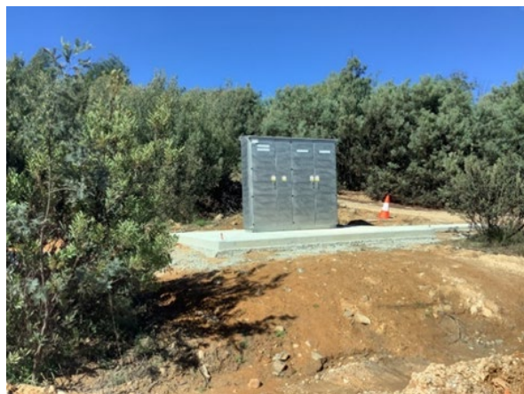
Figure 2 Recently installed 400kV substation
