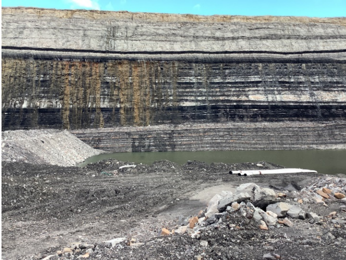
Figure 1 Potential acid mine drainage leachate within the wall of a tailings storage facility
