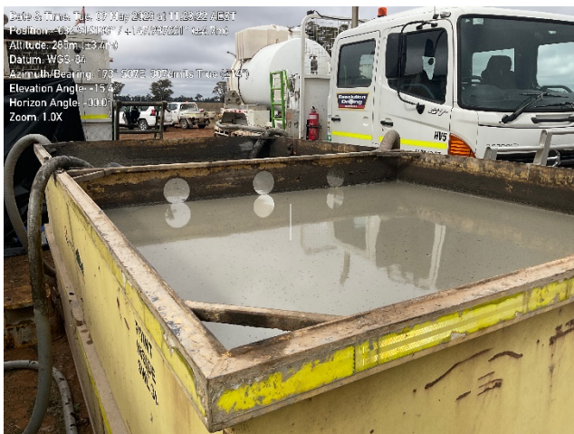
Figure 4 Above ground water management sump
