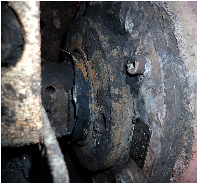
Figure 1: Failed tail pulley bearing
