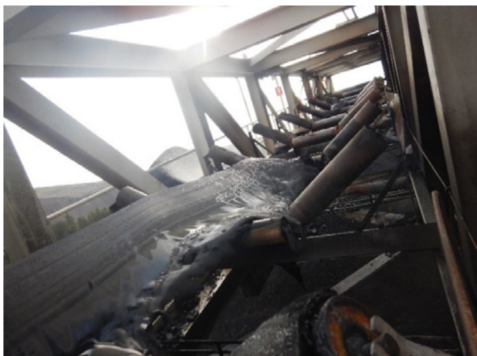
Picture 18. Fire damage to boom conveyor.
