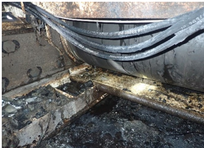
Picture 15. Damage from fire on conveyor pulley.
