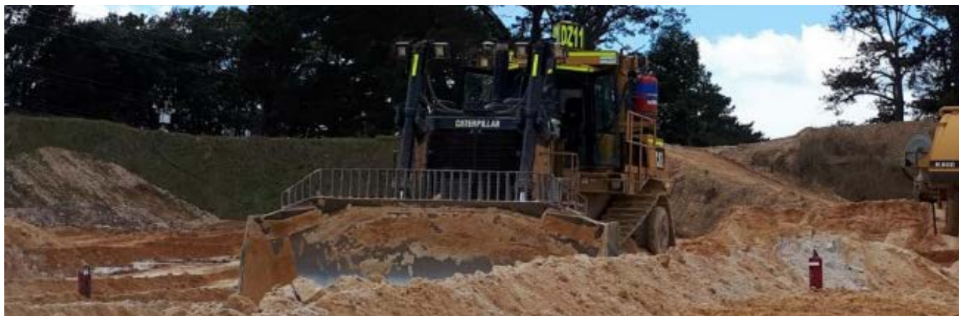
Figure 40 Central Coal Sands Quarry incident
