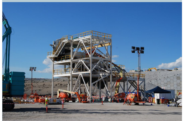
Structure where the accident occurred
