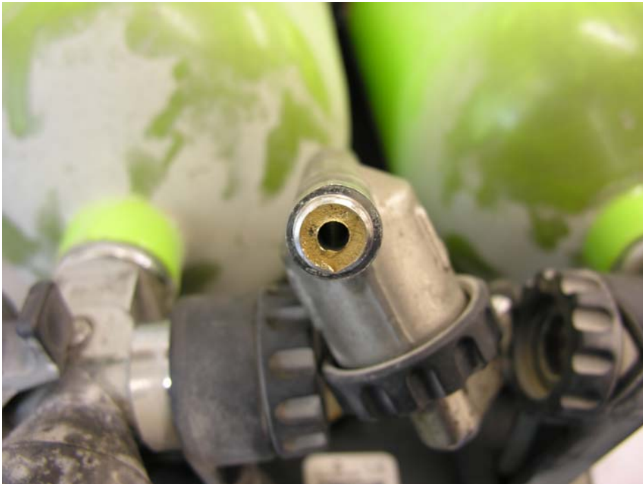
CABA unit showing broken connection
