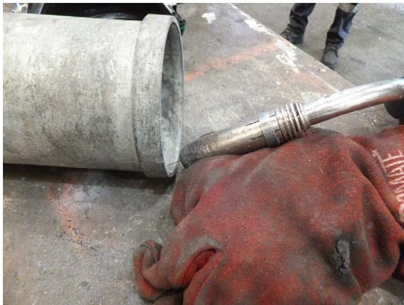
Figure 1: Shock while welding pipe
