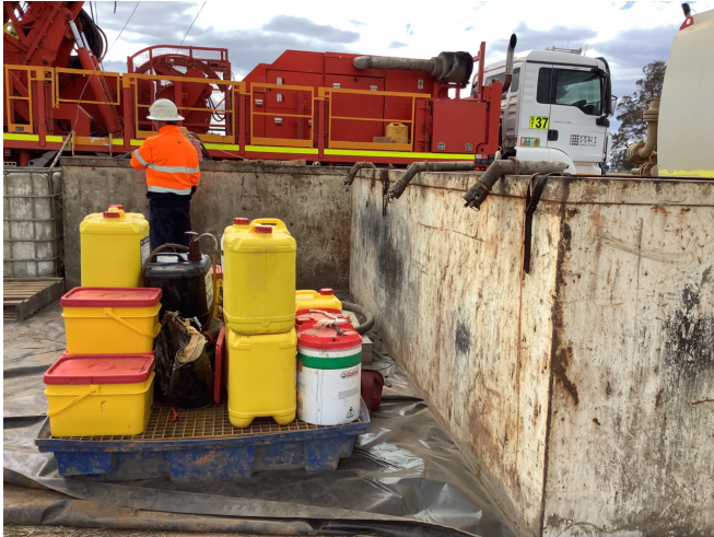
Figure 6 Above ground sumps
