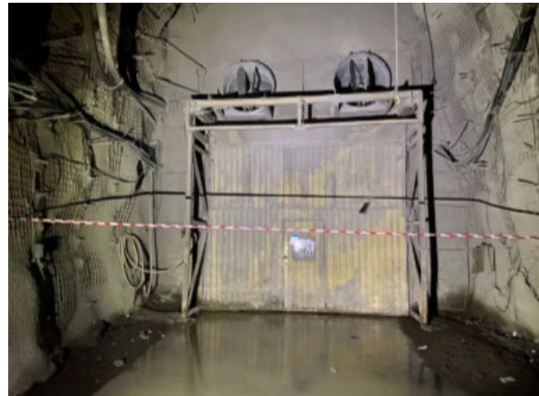
Above: The ventilation door in a closed position.
