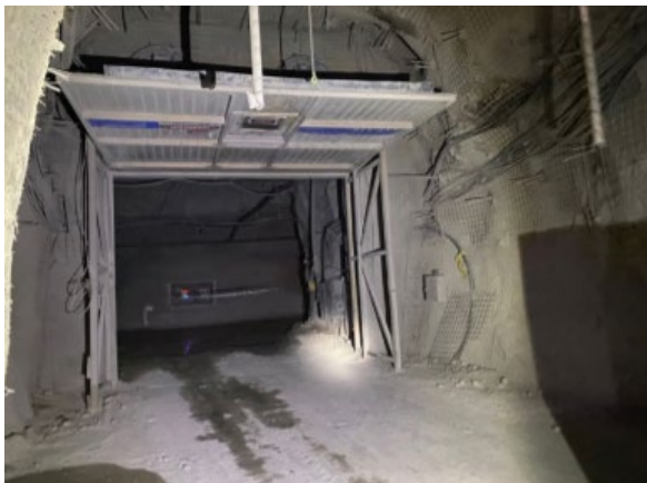
Above: The fully opened ventilation door.
