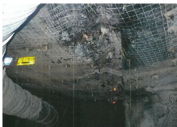
Above: Fallen section, spread across roadway.
