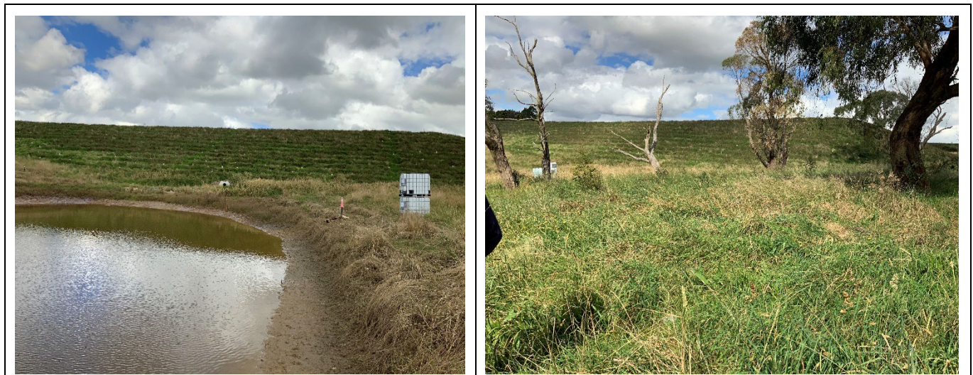
Figures 1 and 2 Northern Visibility Bund in background with evidence of recent planting activity
