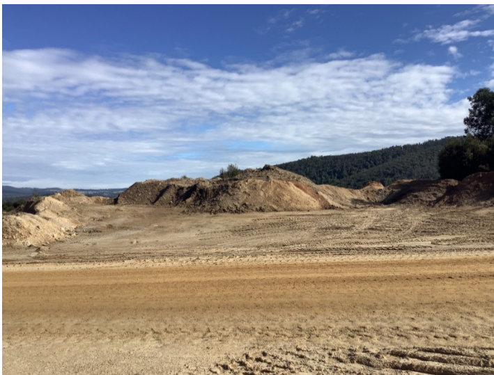
Figure 2 Soil stockpile observed at South-West quarry area
