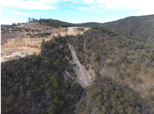
Figure 12 Landslip North-South Quarry bund wall
