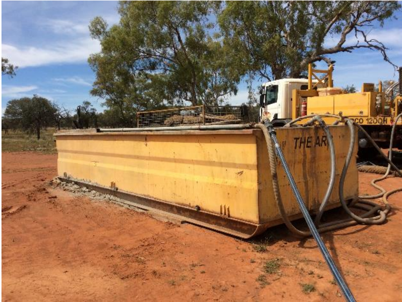
Figure 5 Aboveground sump in use at 20BMDD011
