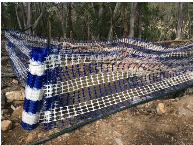
Figure 3 Fenced inground sump at BD20-001
