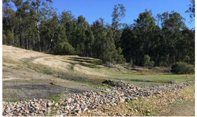
Figure 4 After - waste material stockpiles have been removed and areas seeded to minimise erosion. Rock check dams installed (in the background) slow down flows and capture coarse sediment before run-off collects in the dams
